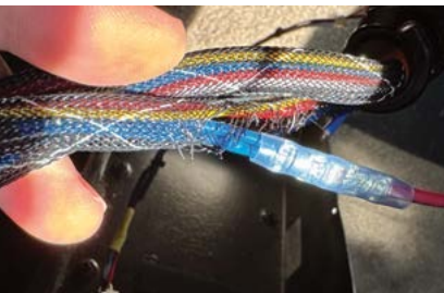
Photo 3: The splice in the relay module harness, bypassing pins 14 and 15
